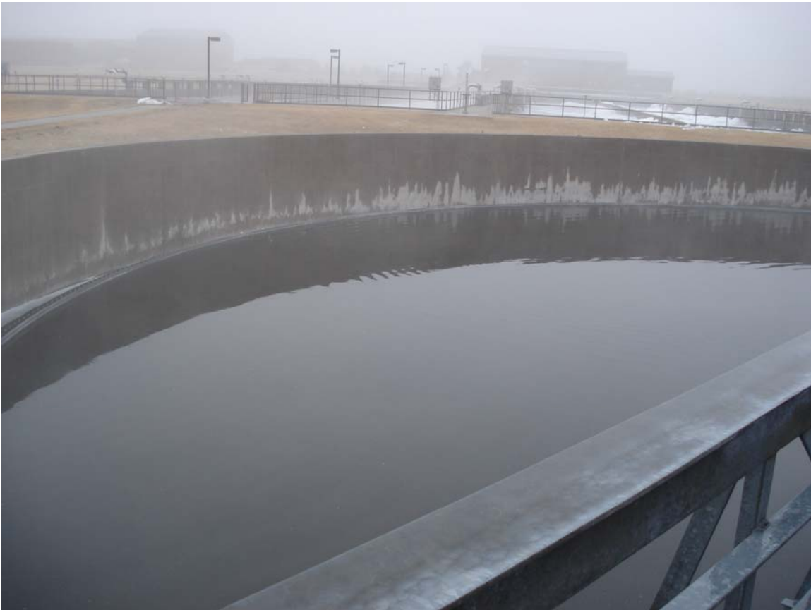
Secondary Clarifier – the water in this is clear enough to see several feet down
