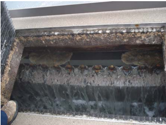
Water flowing out of in- use primary clarifier
