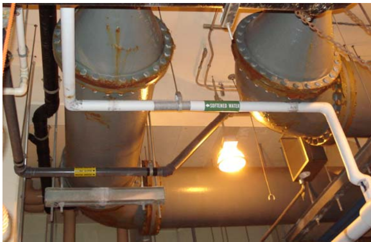
Forced Mains (about 3 feet in diameter)
