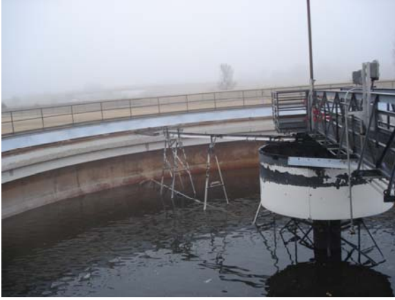
Other primary clarifier – half full and not currently in use (note the metal structure between the upper and lower arm)
