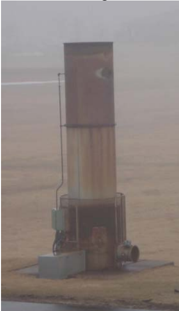
Methane Flare (not currently operating)
